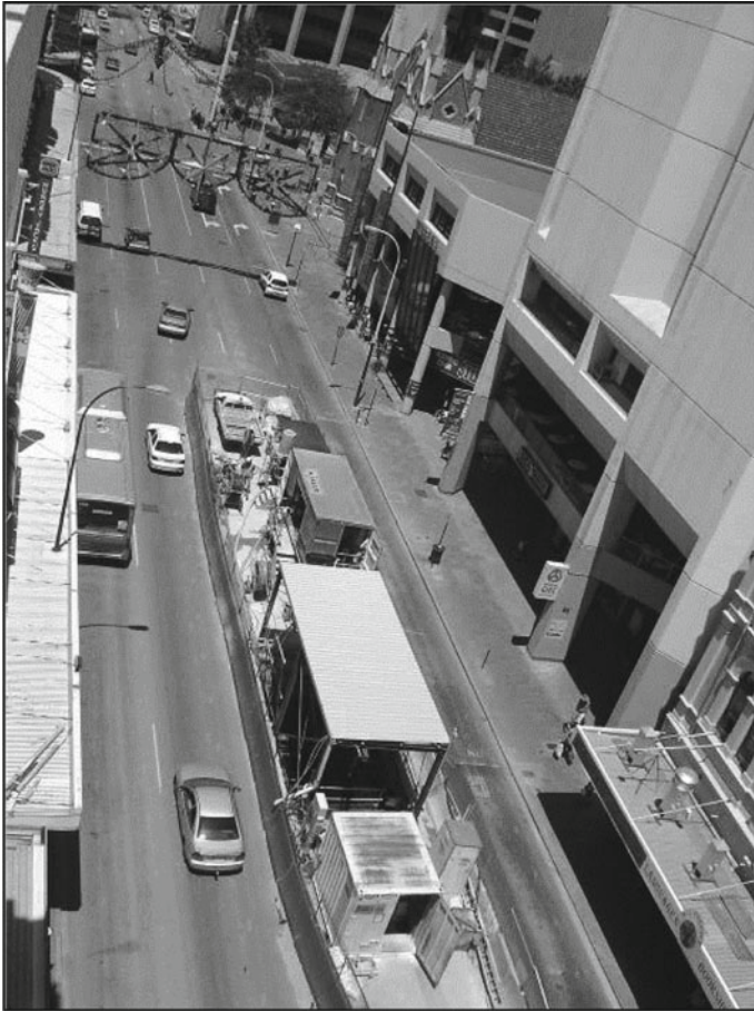
Fig. 5 Access shafts in the middle of William Street. The fan of TAMs spreads from the shaft to the left of the photograph
