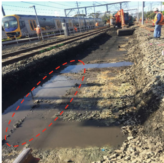
Fig. 1 Mud pumping prone site in New South Wales, Australia
