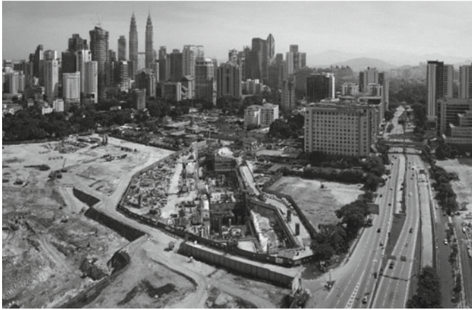
Fig. 12 Ariel photo of Tun Razak Exchange station in construction, after rock fissure grouting
